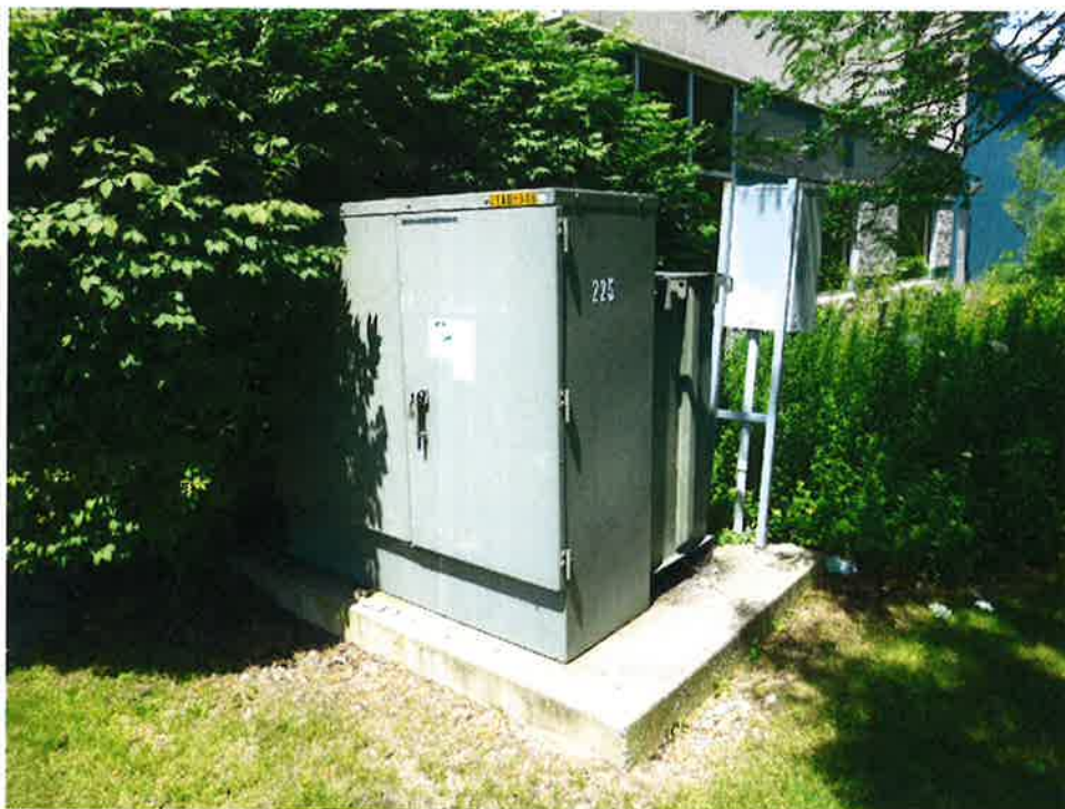
14: View of the pad mounted electrical transformer observed east of the southeast corner of the building on the subject property, facing north.
